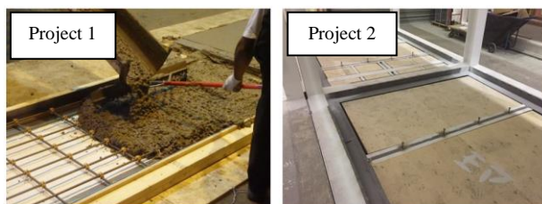
Figure 13. Precast concrete panels to be fit into floor frame in Project 1 (left) compared to formwork fitted in floor frame then pouring concrete directly in Project 2 (right)
