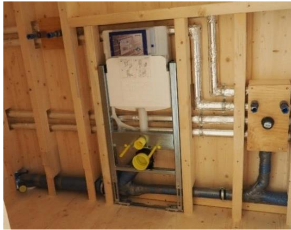
Figure 3. State-of-the-art pipe routing behind a plasterboard wall (room module 9a in Figure 2).
