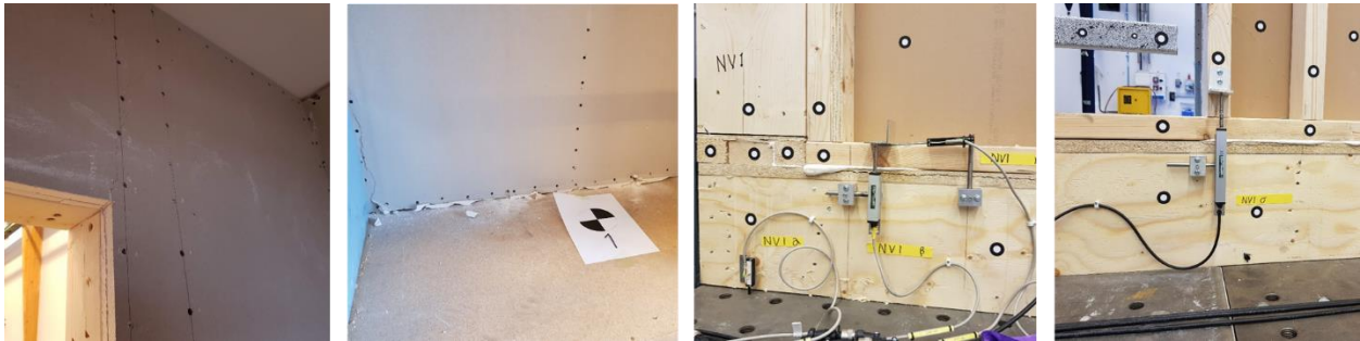
Figure 7. Most visible damage in the gypsum boards and the mechanical connections after unloading of the module.
