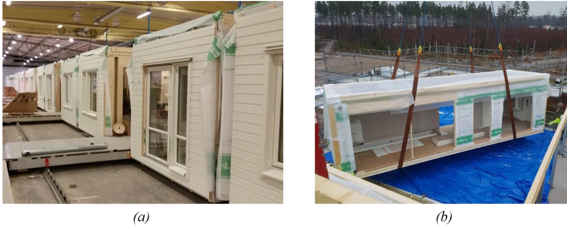
Figure 1. Production of mid-rise modular-based timber building, (a) production of the volume modules in a factory climate, (b) assembly of volume modules on the construction site.
