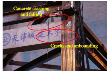
(b) Bottom ceiling beam failure
