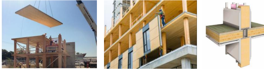
Figure 2. Two-storey mock-up, exterior prefabricated panels being installed and details of the encapsulation of CLT floor (courtesy of Naturallywood.com and Acton Ostry Architects Inc )
